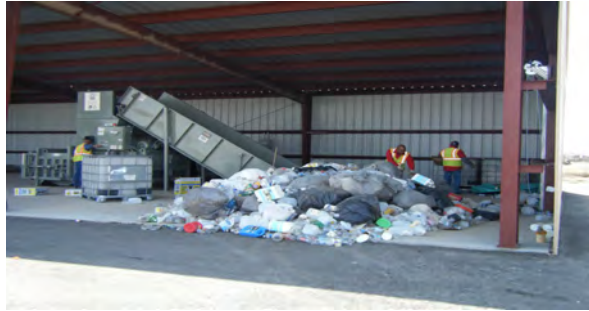
Small Processor: 3,000 square foot processing facility, capable of processing about 4 tons per day.
